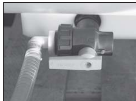
Tank valve positioned for liquid-flow (open) to pump.
