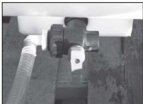
Tank valve in Off position for cleaning filter.
