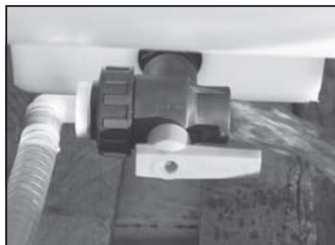
Tank valve in drain position.
