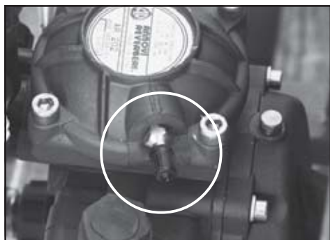
Check pressure in pump air chamber regularly.
