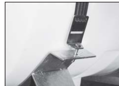
Make sure tank straps are tight.
